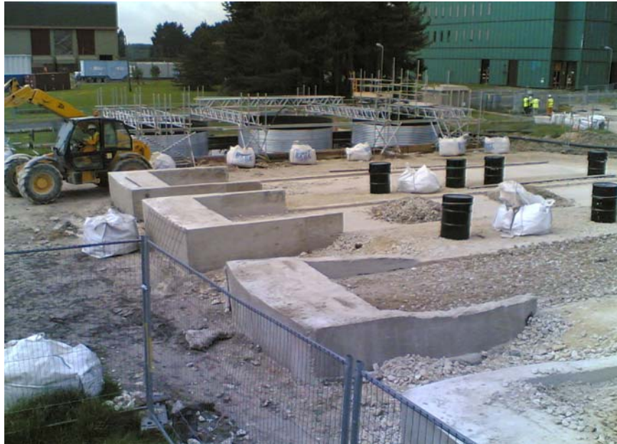
Figure 4: Monitoring of concrete debris in the external troughs with LLW drums ready for removed materials with dewatering tanks in the background.
