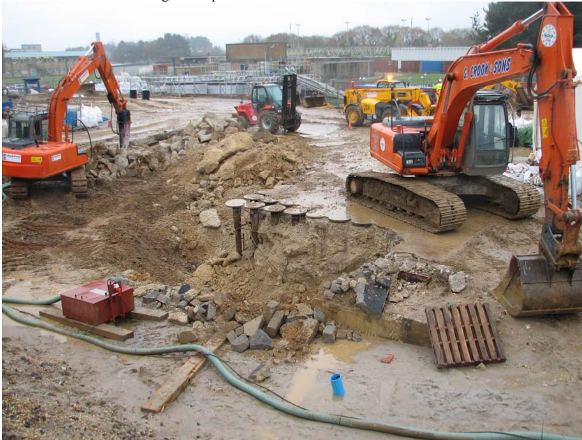
Figure 3: Recovery of deep mortuary tubes from base slab close to dewatering well
