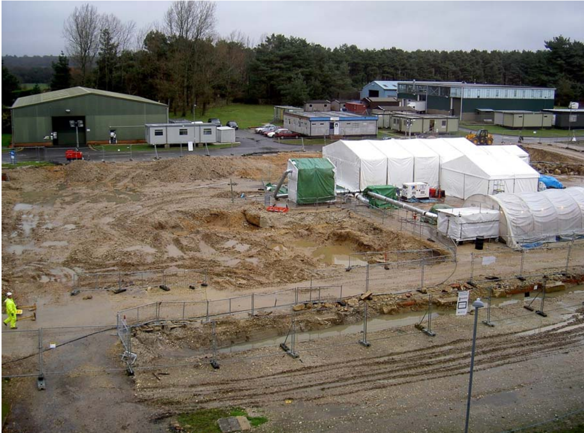
Figure 2: Ventilated Enclosures over NCL and Decontamination Bay Sump Areas also showing the Zone 1 area cleared of concrete to left side. Note also the presence of groundwater in puddles after rain due to clay content of the soil
